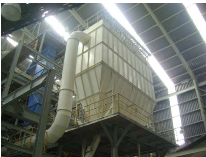
Figure 2. New dedusting system within a compaction-granulation unit.
